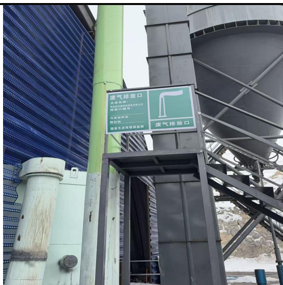
破碎粉尘排气筒标志标牌
